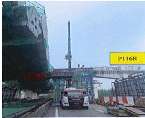
Figure 1. Condition before accident
