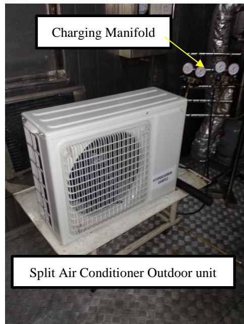
Figure 2: Outdoor unit undergoing test in psychrometric chamber.
